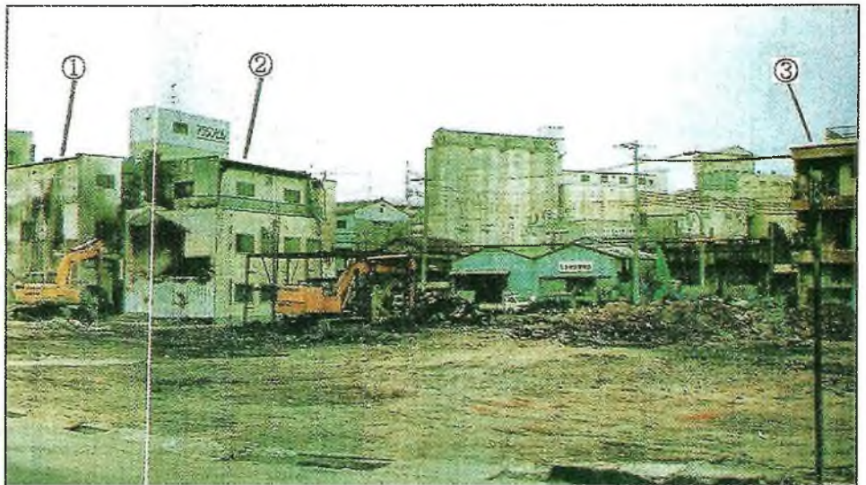
Building 3 ALC Structure is still standing even with gutted interior. ALC 1 & 2 are intact.
