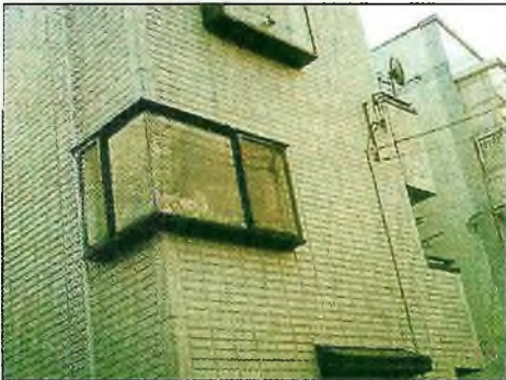
ALC building with Tiled ALC exterior wall : degree A
